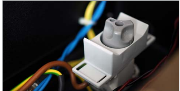
Heavy-duty circuit breaker inside the PSU.
